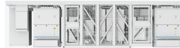
Delta 7.1MVA SKID Switchgear+MV Transformer +2*PCS 3556kW
